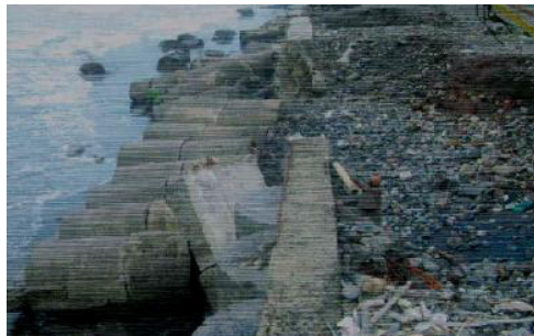
Figure2. The damageson the seawall south Pasauran beach (Junarsa, 2006)
